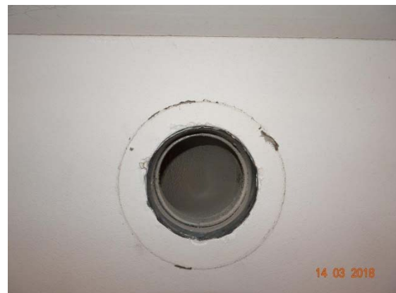
Abbildung 195: WNG ID 820: ABL-Rohr, Bad
