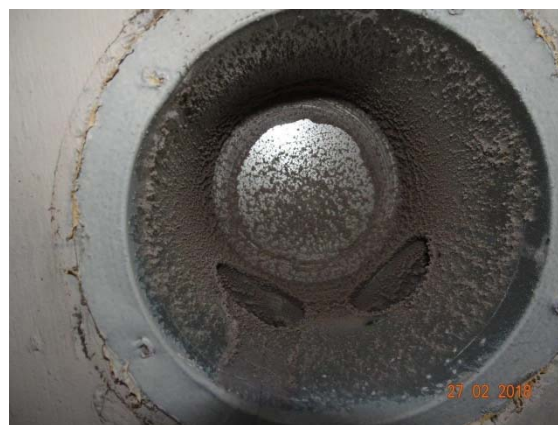
Abbildung 161: WNG ID 720: ABL-Rohr, Bad
