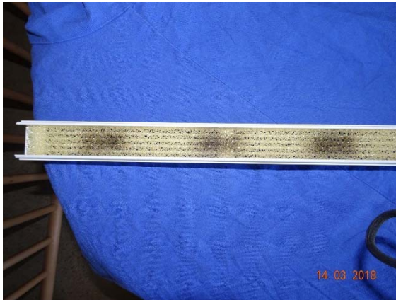
Abbildung 185: WNG ID 810: Zuluftfilter.
