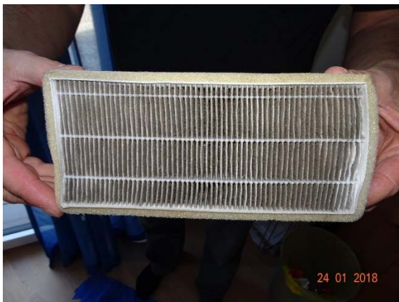
Abbildung 136: WNG ID 620: Zuluftfilter
